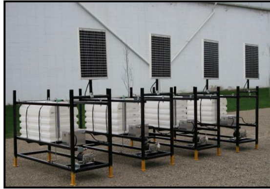
Solar Pump Packages with Various Tank Sizes
